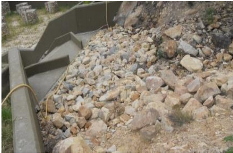
Plate 1 - Loose Surface Materials at Debris Approaching Zone
